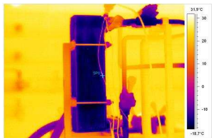
Picture 5.12: Thermographic picture of the plate heat exchanger during unstable operation
