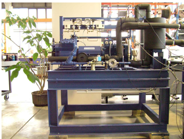
Figure 4.19: View brine chiller
